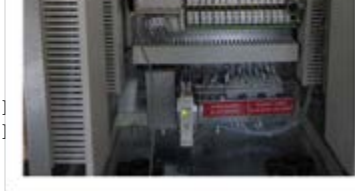
Fig. 13. Integration of control logic within 36-kV GIS.
