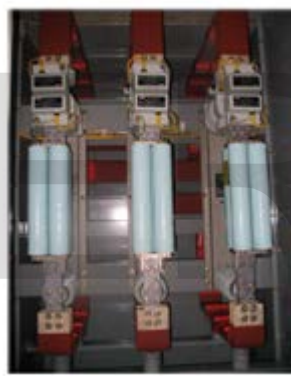
Fig. 2. 15.5-kV 3000-A FCL installed in offshore lineup.
